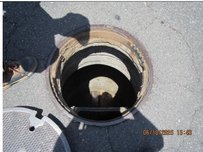
Photo 22: Cracking in the concrete around the manhole.
