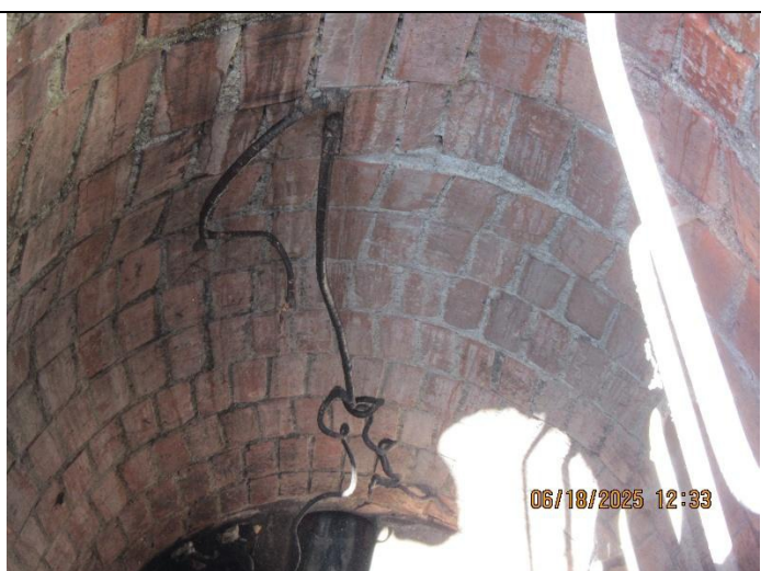
Photo 9: Large roots growing into barrel.
