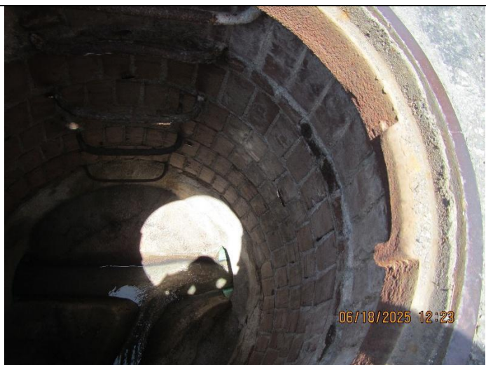
Photo 7: Minor rust visible on the manhole rim.
