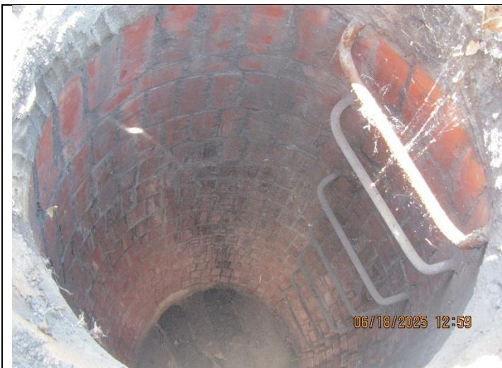
Photo 14: Upstream brick manhole of siphon. Cobwebs and rusted steps visible.
