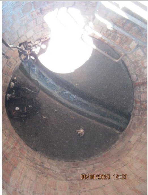
Photo 11: Debris on bench, fast flow through channel, and roots growing into barrel.
