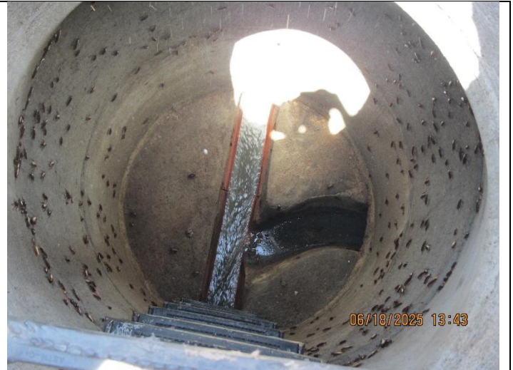
Photo 21: A significant number of cockroaches visible. Fast flow through the mainline, but some feces built up in lateral with standing wastewater.
