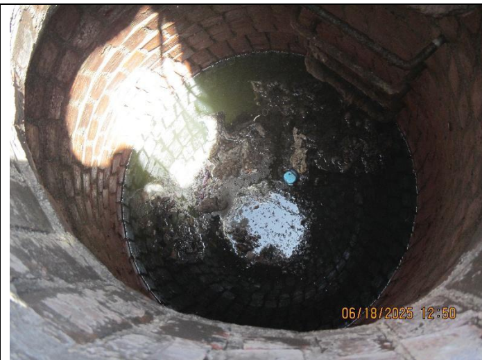
Photo 13: Bench and channel not visible as bottom of manhole filled with wastewater, solids, and trash.
