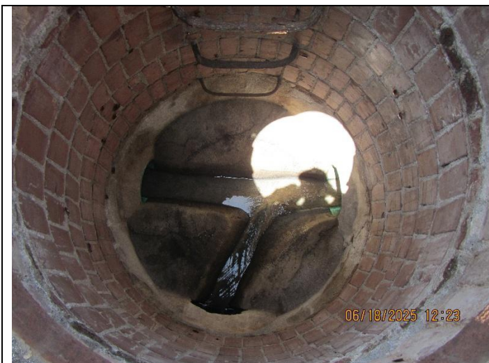
Photo 6: View inside the brick manhole showing two incoming pipes and one outgoing pipe. Mortar appeared to be in decent condition and there was no debris on the bench.
