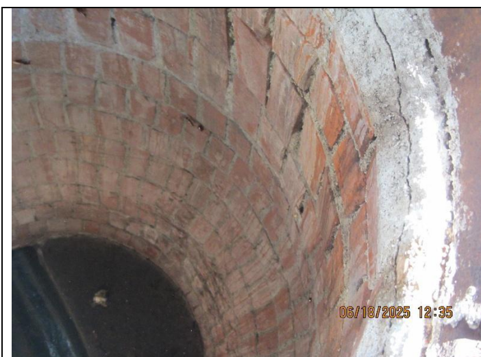
Photo 8: Close-up view of brick manhole showing gaps between the bricks due to eroded grout.
