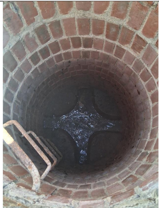
Photo 24: View inside the brick manhole showing rusted steps, mortar in okay condition, and good flow through the channel.
