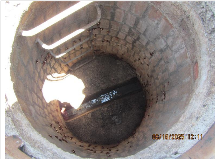
Photo 3: View inside brick manhole showing mortar in good condition, minor flow, and cockroaches in barrel.
