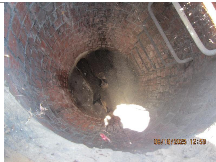
Photo 15: Bench is eroded with missing pieces. Dirt and debris on the bench and no active flow through the channel.
