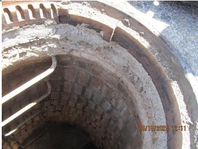
Photo 5: Photo showing minor deterioration in upper barrel.
