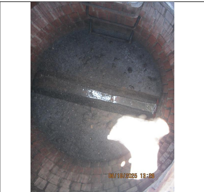
Photo 19: Staining in the barrel and debris on bench visible.
