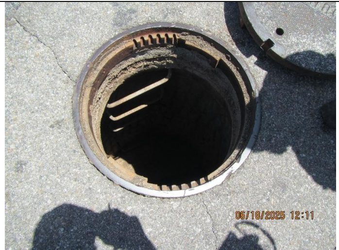
Photo 4: Cracking in concrete around manhole and minor rust around rim.
