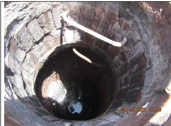
Photo 12: Downstream brick manhole of siphon. Rust visible on steps and around manhole rim.
