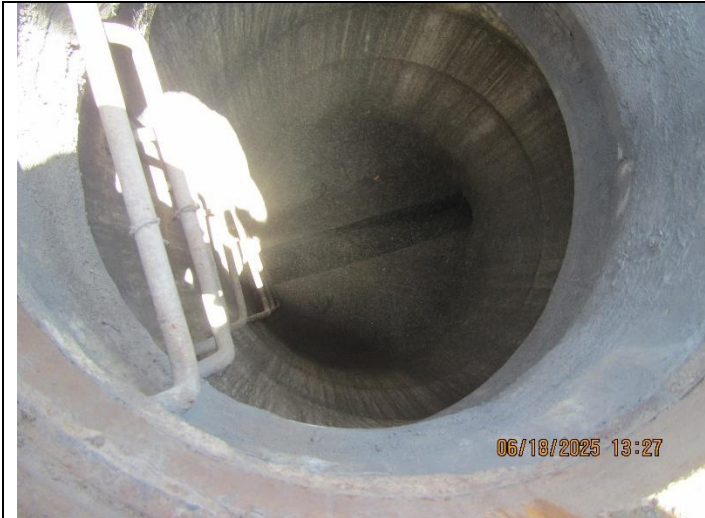
Photo 16: Upstream concrete manhole with staining in the barrel.
