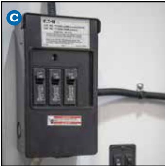
Electrical Panel Box
